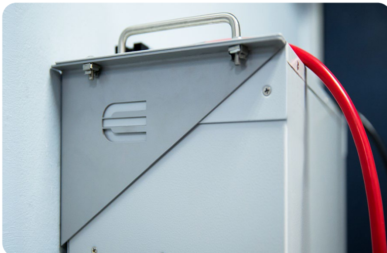
Figure 4: eTower 2 Mounted on the Wall Mount Bracket
