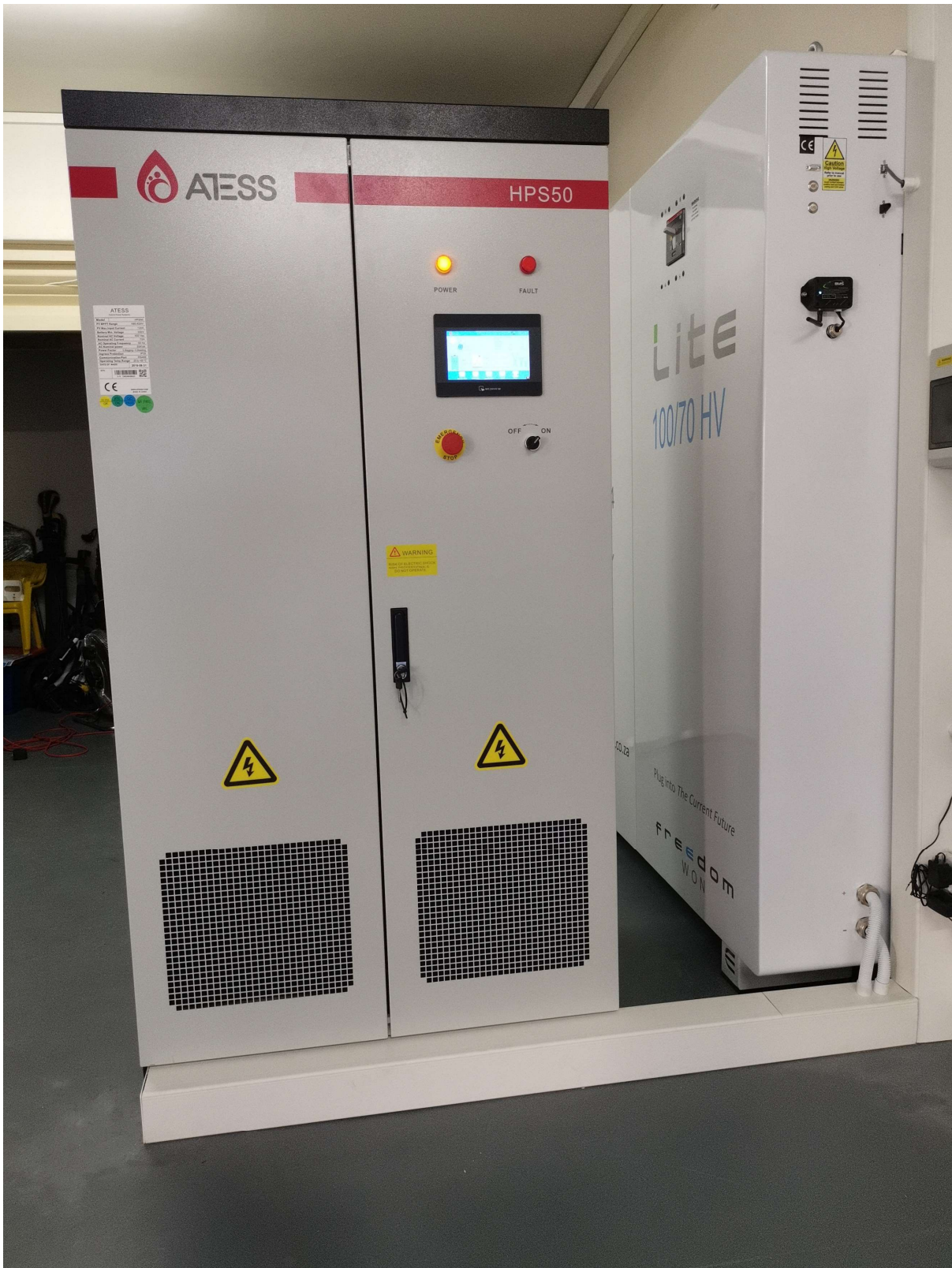
Fig 2.3 Installation Example of a Lite Commercial 100/70HV (now 100/80) with a ATESS HPS50 and no cable trench (trunking used instead)
