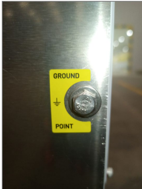
Figure 5: Grounding Point Example
